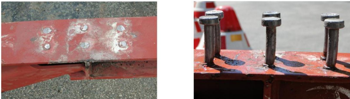
Figure 4. Shear failure of connectors at the edge zone and in less stressed interior span area.
